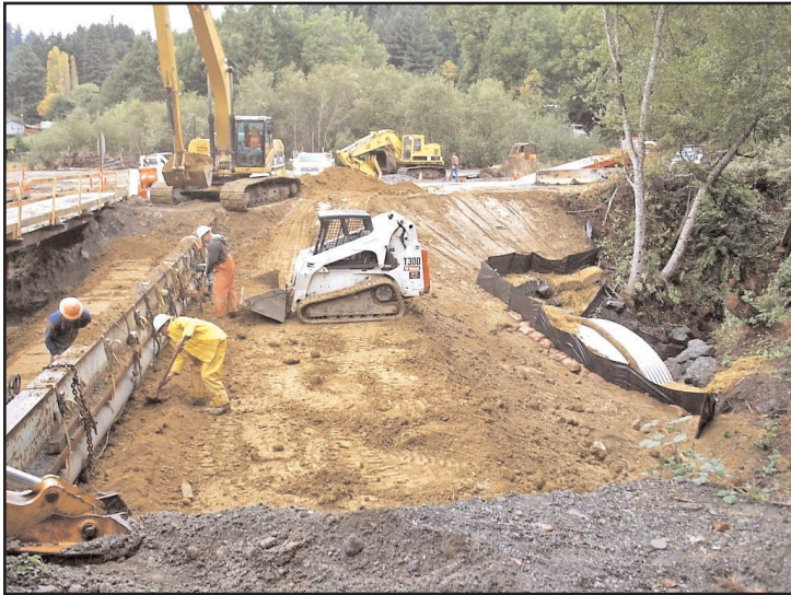
Restoration of degraded watersheds, such as placing a culvert in Humboldt County's Warren Creek, is a primary goal of A.B. 2575.
